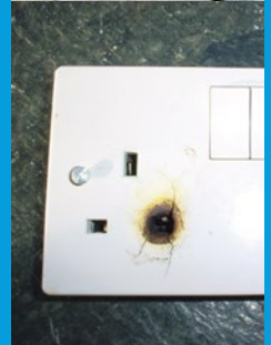
Typical examples of potentially dangerous electrical installations
